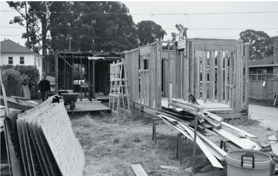
Reusable materials are sorted as they are removed from this Santa Cruz deconstruction site. Photo courtesy of Deconstruction Industries, Inc.
